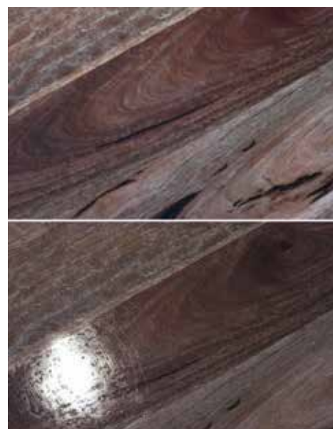
The same area of flooring but with down lights on in the lower photo. Down lights highlight sanding imperfections and dust, some of which can be acceptable.
