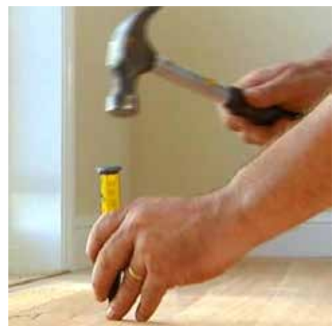
Nails to be punched and holes filled.
