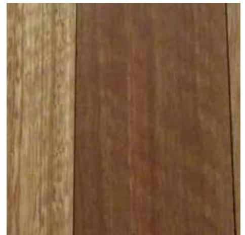
Small gaps at board edges may occur, particularly during dry weather.
