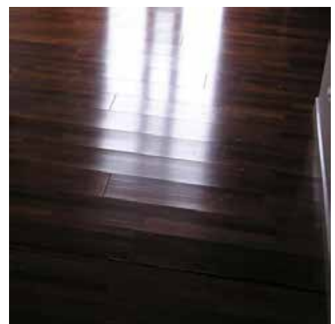
Peaking due to expansion pressure
