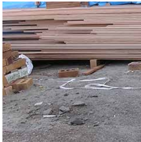
Inappropriate site storage that can void manufacturer warranties.
