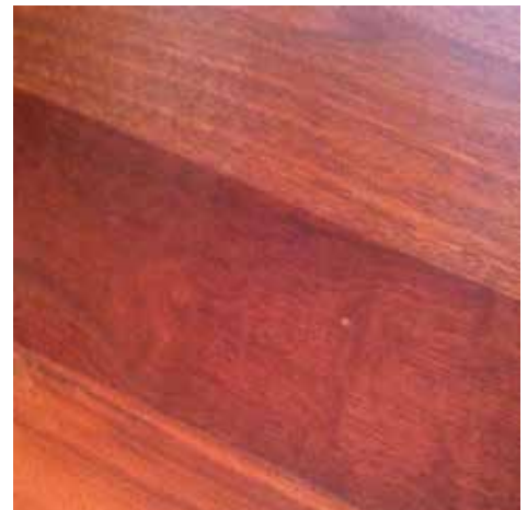
The nail penetration is to the right of centre in the photo
